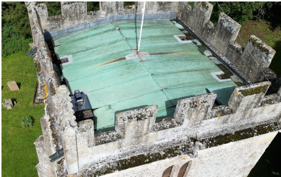
Figure 4 – Tower roof – consider renewing in lead.
