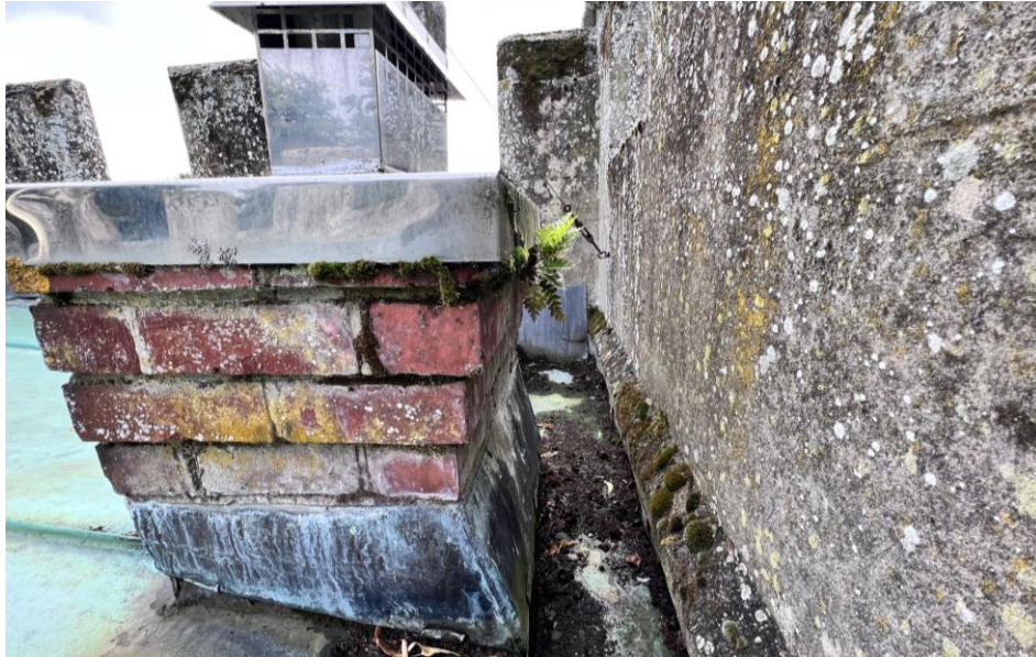
Figure 5 – Tower roof, chimney – remove plant growth.
