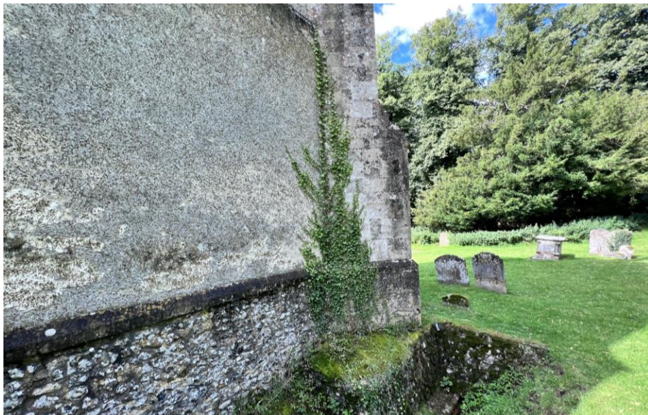
Figure 18 – Tower, north west buttress – remove ivy.
