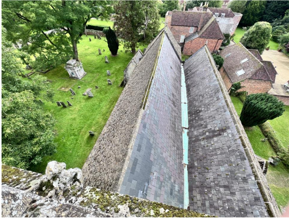
Figure 7 – Nave and south aisle roof – reinstate slipped slates.
