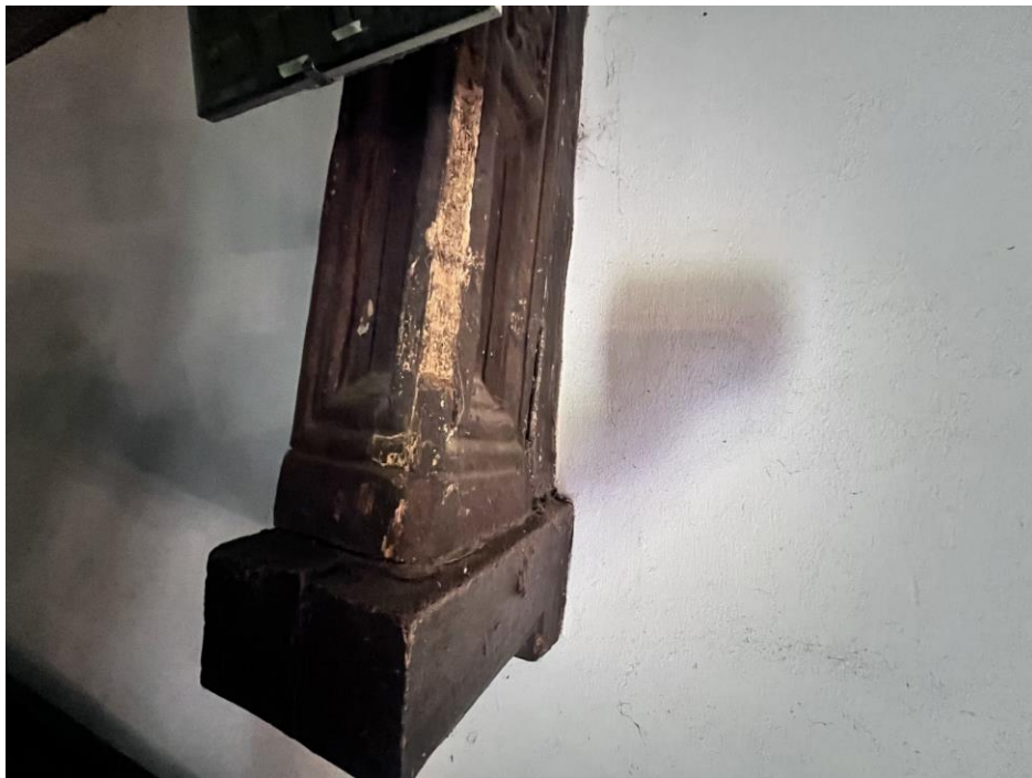
Figure 30 – Nave roof wall post – treat beetle attack.
