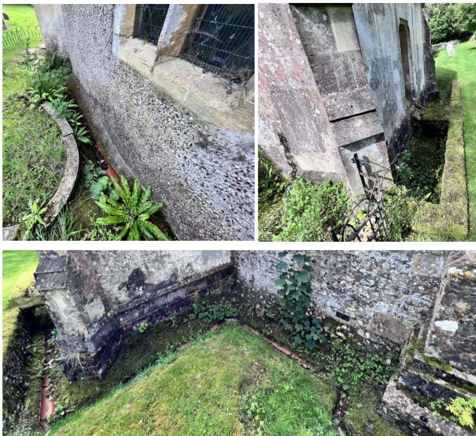
Figure 16 – Perimeter drainage channel – clear plant growth.
