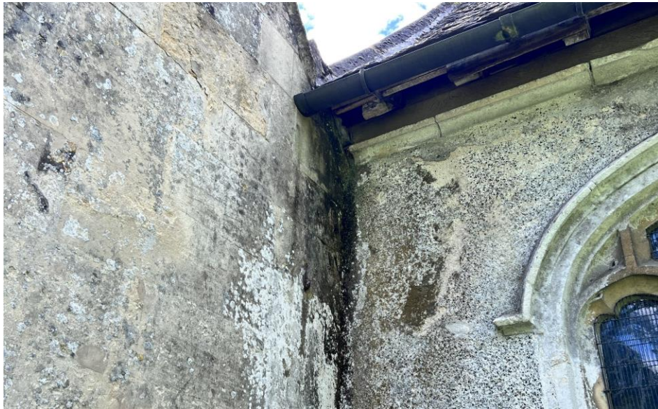
Figure 11 – Nave, north – investigate overflowing gutter.
