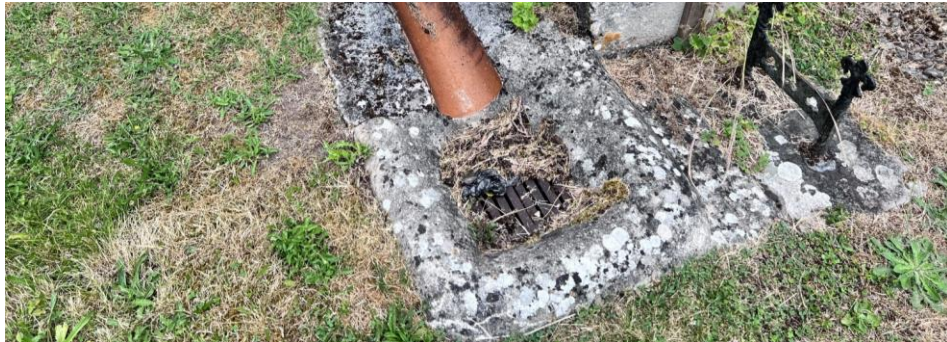
Figure 15 – Porch – clear gullies.
