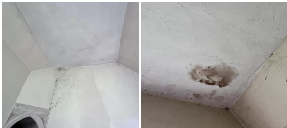
Figure 36 – Vestry – ceiling may need renewing.
