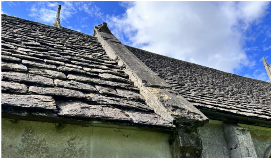
Figure 9 – Vestry roof – repair/replace damaged copings.
