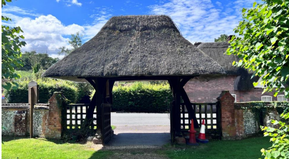
Figure 43 – Lychgate – repair/replace rotten timbers, remove ivy, renew thatch.
